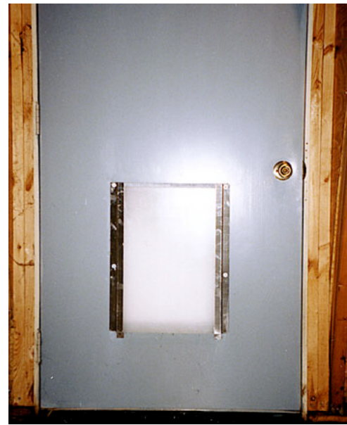
An installed closure on metal door Photo 2
