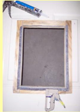
Use silicone caulking around trim kit for add insulation. To quiet door
